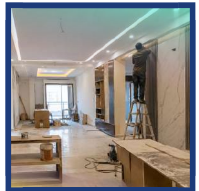
False Ceiling & Lighting
